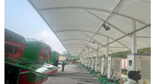
Charging Stations – Telangana
