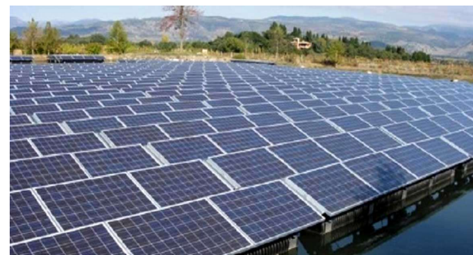
Feeder Solarization Project, Maharashtra
